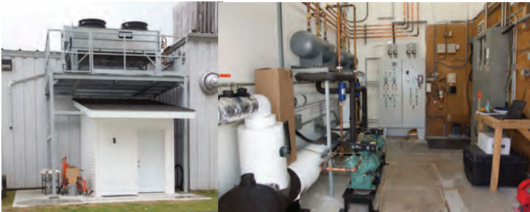
New ice plant exterior and interior mechanical room
